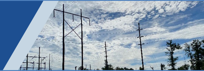
Photo by Tunis Substation
